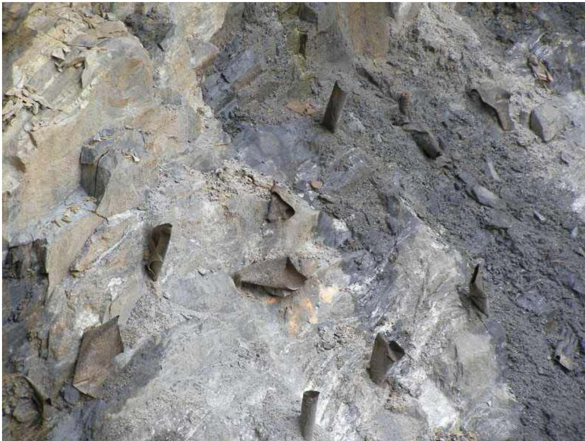
Photo 9 – Marks of Drillings
