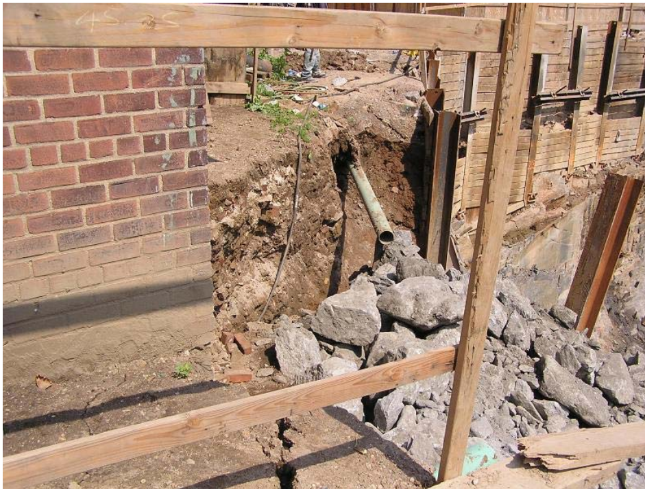
Photo 11 – Broken drainage pipe at collapse area
