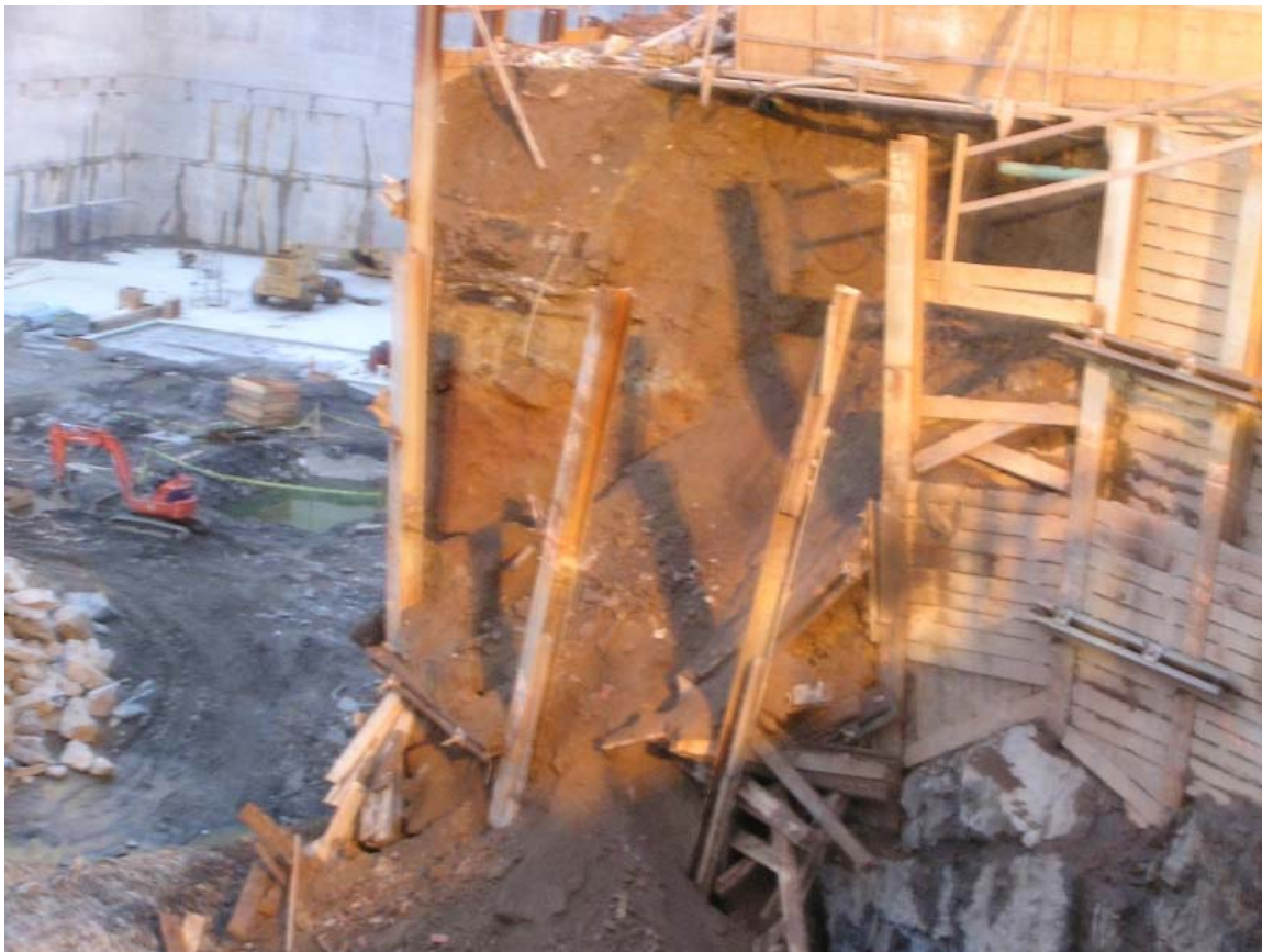
Photo 1 – The Collapsed Sheeting
